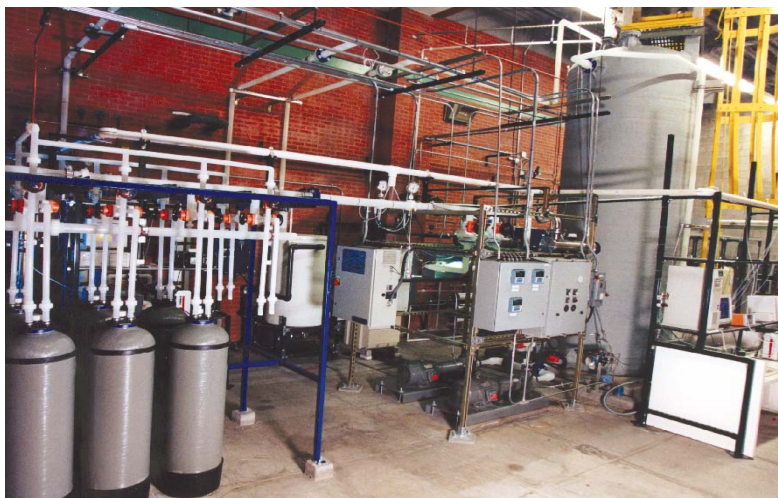
This state-of-the-art, ultrapure water system delivers water of part-per-billion purity levels for research in wafer cleaning, ultrathin oxide growth, and advanced chemical-mechanical planarization research and post-CMP cleaning techniques.
